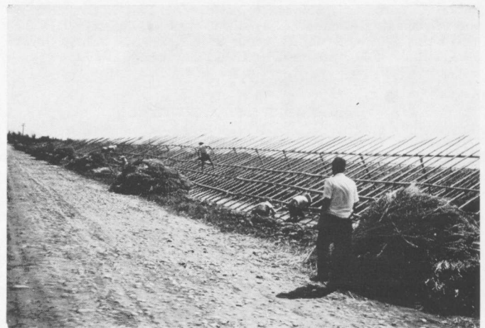
Workers are constructing a framework of bamboo poles over which is placed a layer of rice straw. When completed, this structure provides an effective windbreak and reduces fish mortality in wintering ponds.
