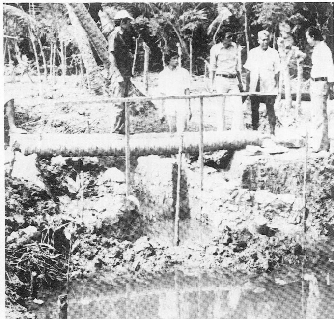
A fish farmer receives technical assistance from his area extension agent and the BFP project supervisor during construction of a new concrete water gate for his tambak. Project staff made more than 10,000 individual farm visits to fish farmers in Aceh and North Sumatra between 1976 and 1978.
