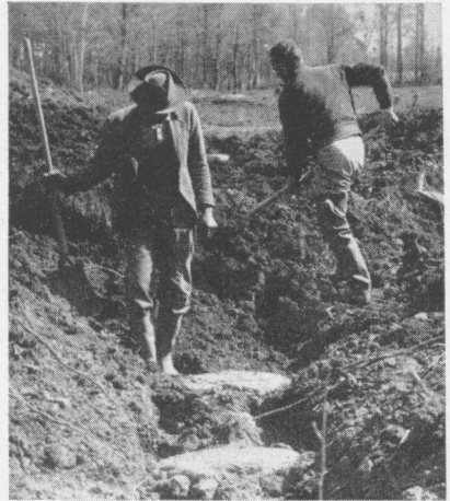
FIG. 21. As soon as the joints are poured, they are covered with thin layers of clay. The clay is then applied along each side of pipe. It is wet and well packed to a height of 4 or more feet over pipe before concrete hardens.
