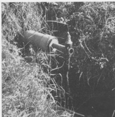
FIG. 36. A pipe with a valve is used for controlling the water entering the pond through the diversion dam.
