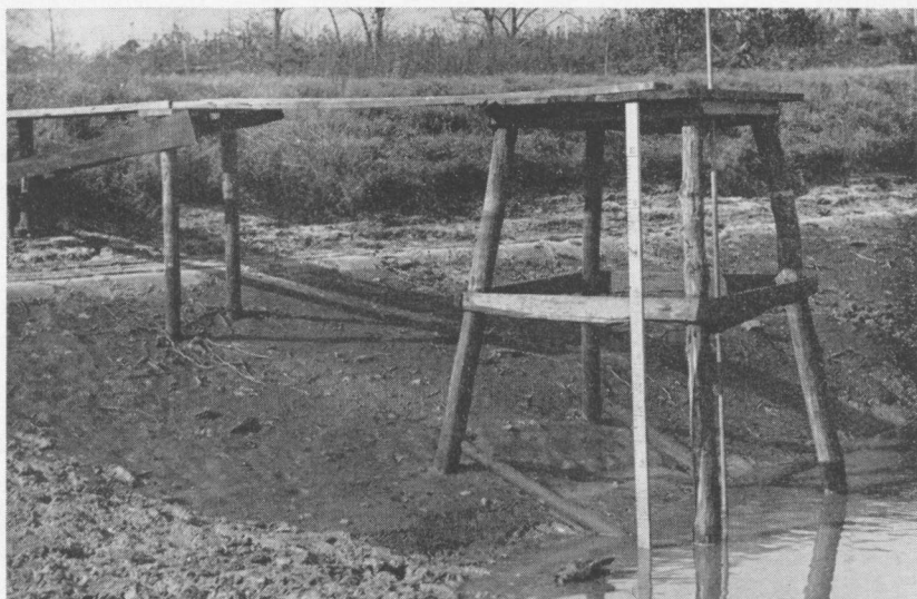
FIGURE 26. Shown here is a wood platform from which the gate valve is operated. Untreated wood is not satisfactory because it rots within 5 years. Pressure-treated, creosote posts or concrete posts are recommended.
