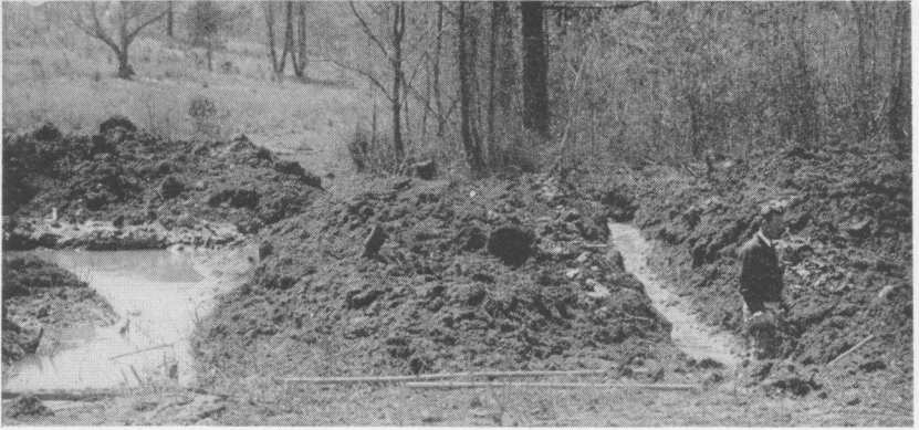
FIGURE 16. Shown here is base of the dam that has been built to a height of 4 feet above the stream, which is being diverted on the left. The ditch for installing the drain pipe has been dug across fill on the right.
