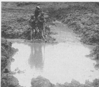
FIG. 14. Shown in foreground is a portion of the trench that has been blasted a second time. The men are loading dynamite to complete the second line of charge.
