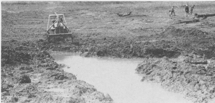
FIGURE 15. All undesirable materials have been blasted from trench in the boggy area. The tractor is now starting to cut the trench on the hillside. This good clay is used to fill the trench across the bottom.
