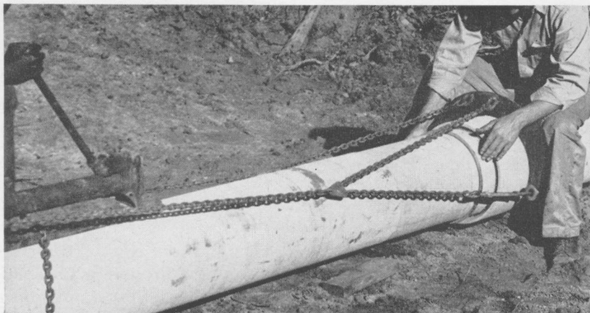
FIGURE 19. A hydraulic jack assembly, as shown, is used to pull the collar in place over the rubber ring to seal the joint of asbestos-cement pipe.
