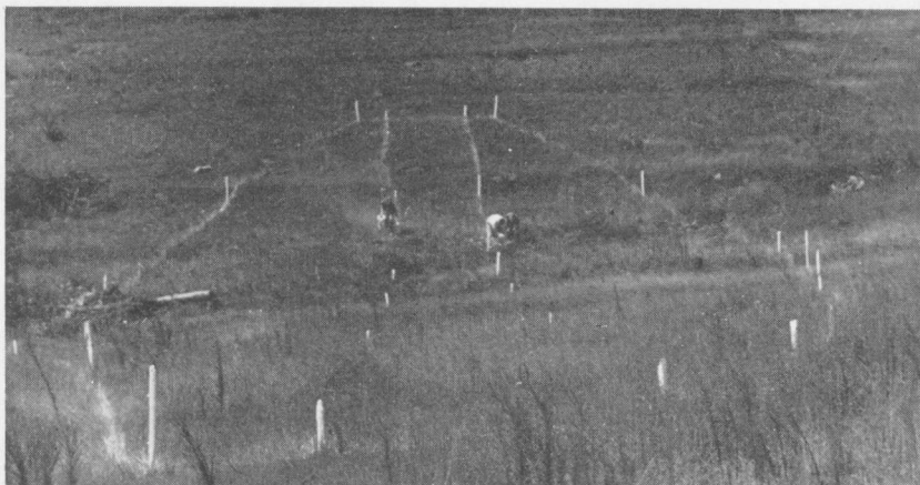
FIGURE 3. In the layout of proposed base of dam shown here, the two straight lines of stakes across the hollow outline the width of top of the dam when it is completed. The outside rows of stakes (toe-stakes) outline the area that the base of the dam will cover.
