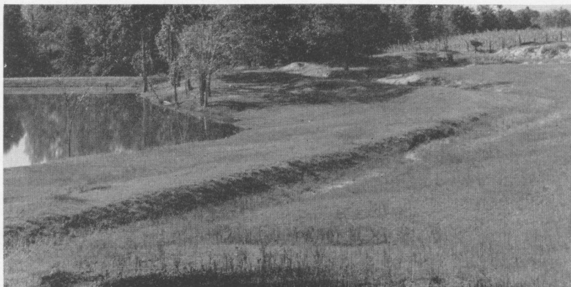
FIGURE 35. A diversion ditch is built on hillside to by-pass excess water around the pond. This ditch is sodded to prevent erosion.
