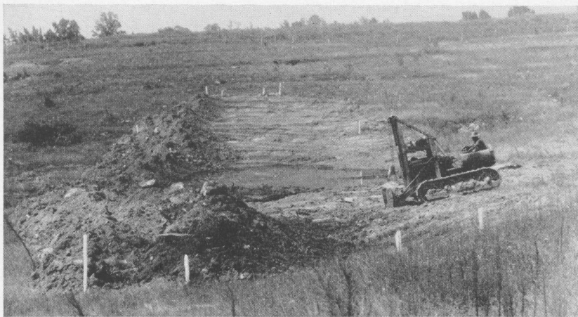
FIGURE 8. Tractor with bulldozer attachment pushes topsoil from base of the dam to the downstream toe. This operation is done prior to cutting the core trench.
