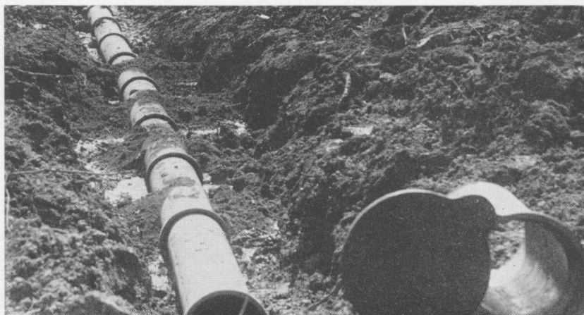
FIGURE 18. Joints of cast iron soil pipe are laid in the ditch. Here the line is being straightened and held in place with dirt preparatory to caulking and concreting the joints. The flap valve at the right will be placed later in the bell joint of the drain pipe in foreground.
