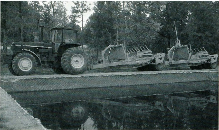
Figure 8. Earth-moving equipment used in the construction of levee catfish production ponds. This equipment is fitted with a laser leveling instrument to allow precise placement of clay on the dam.
