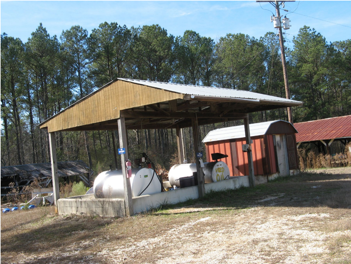
Figure 63. Fuel storage facility installed on the old Field Headquarters site on the Story Farm. Note that the abandoned 'Saw Mill' shed is shown in the background in the lower left-hand corner.
