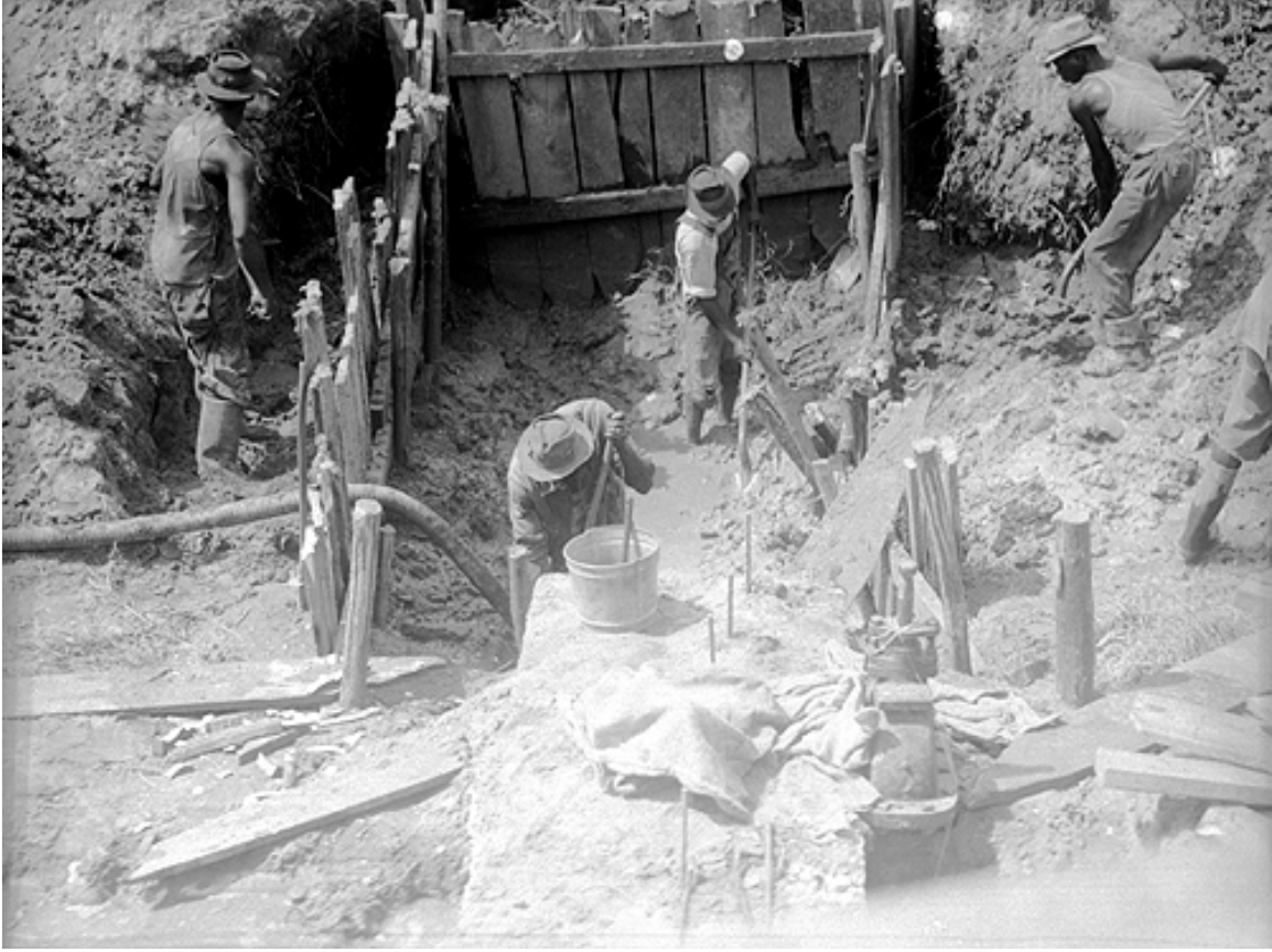
Figure 20. Construction of the 'low-head' dam on Funchess Creek. The small reservoir created by the construction of the dam raised the water level of the creek so that it would flow into the diversion ditch, supplying water to for the 'E,' 'F' and 'M' Ponds.
