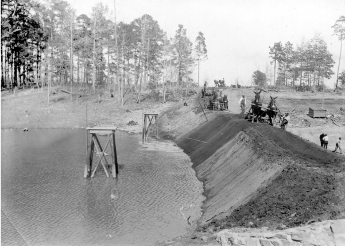
Figure 7. Using mules and 'slip-scrapes' to complete the Farm Pond 1 dam. Picture was taken from the south. East University Drive would later be located on the 'brow' of the hill to the north. Note the galvanized water supply pipe protruding from the dam. Also note the steel rod attached to the 'pier' in the foreground. This rod was used to open and close the 'flap' valve employed in draining and filling the pond.
