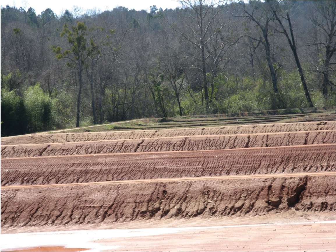
Figure 61. View of several of the re-constructed 'E' Ponds. Forest along Soughahatchee Creek is in the background. These ponds will be part of the 'B' Series (B-5, 6, 7 and 8).
