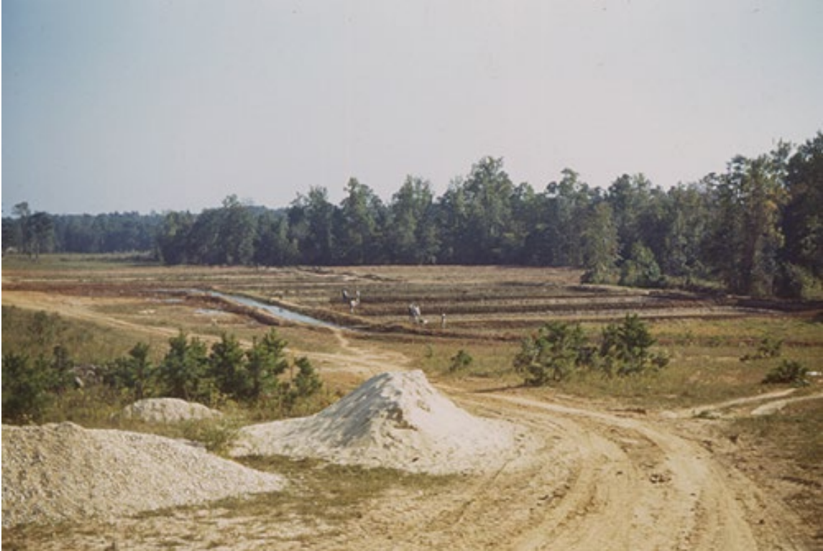
Figure 21. View of the 'F' Series construction site in 1940. View is from north to south. Soughahatchee Creek is at the far south end of the clearing. The small dam has been completed on Funchess Creek, to the extreme right. Water from the small impoundment is flowing through the diversion ditch in the foreground. Ponds F-1 through F-15 are filling. Core trenches for the dams on the remainder of the Series are being dug and filled with heavy clay.
